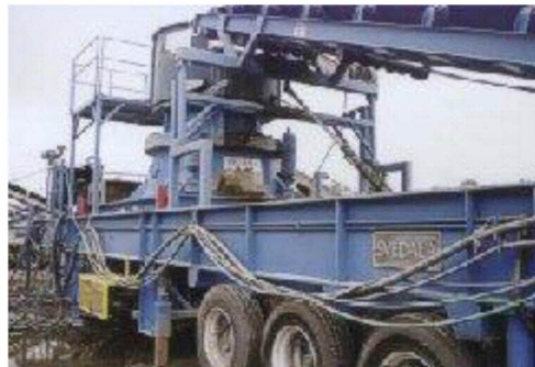
Svedala H6000 Hydrocone operating as the secondary crusher for plant No. 1.
