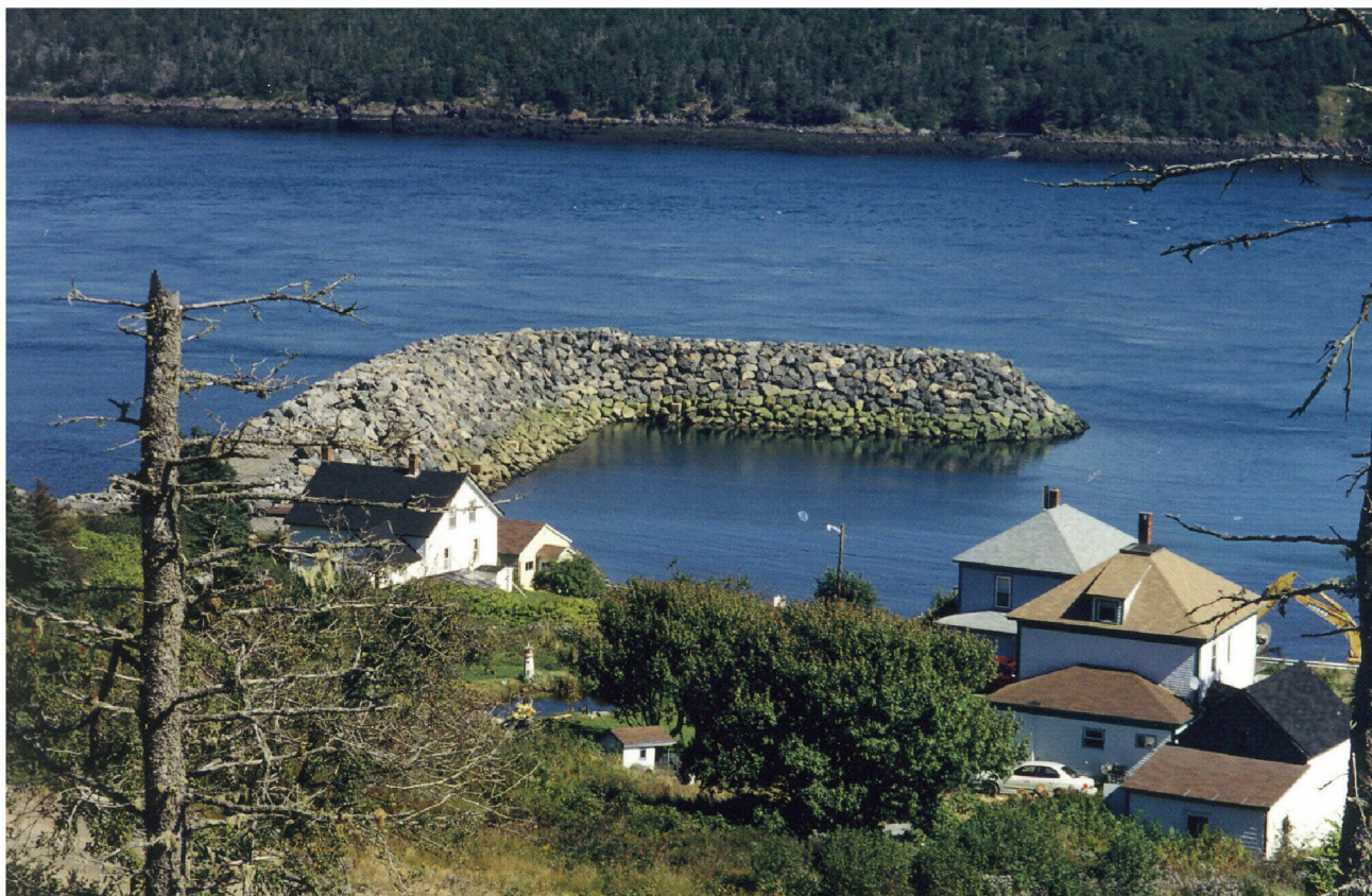
Figure 9. A recently constructed breakwater made from basalt armourstone at Tiverton, Digby County.
