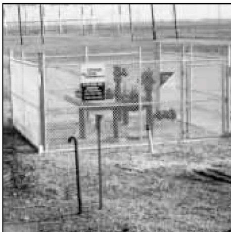
Figure 13. Photograph of a Typical Mainline Valve Station
