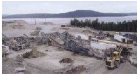
Layout of plant No. 2 with a Cat 988F feeding a Svedala 32x42 primary jaw crusher.
