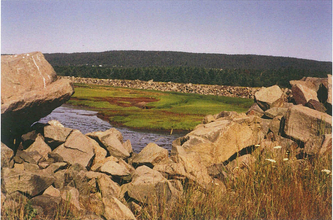
Figure 10. Basalt armourstone used to protect a dyke from erosion at the head of St. Marys Bay near Roxville, Digby County.
