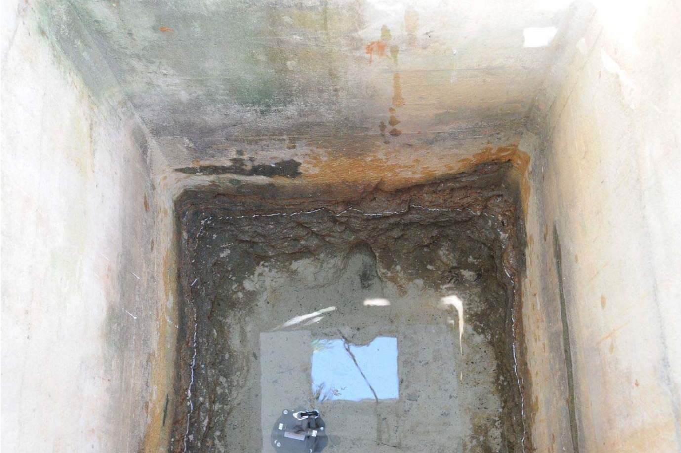
Well on Taiping Island
