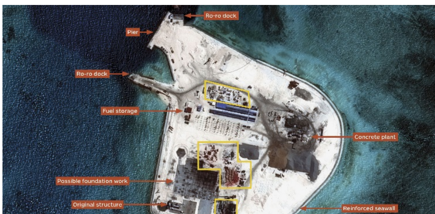
Satellite imagery dated 14 August 2014 shows ongoing construction and development of the new island on Johnson South Reef in the Spratly Islands. (PLEIADES © CNES 2014, Distribution Airbus DS / Spot Image S.A. / IHS)
