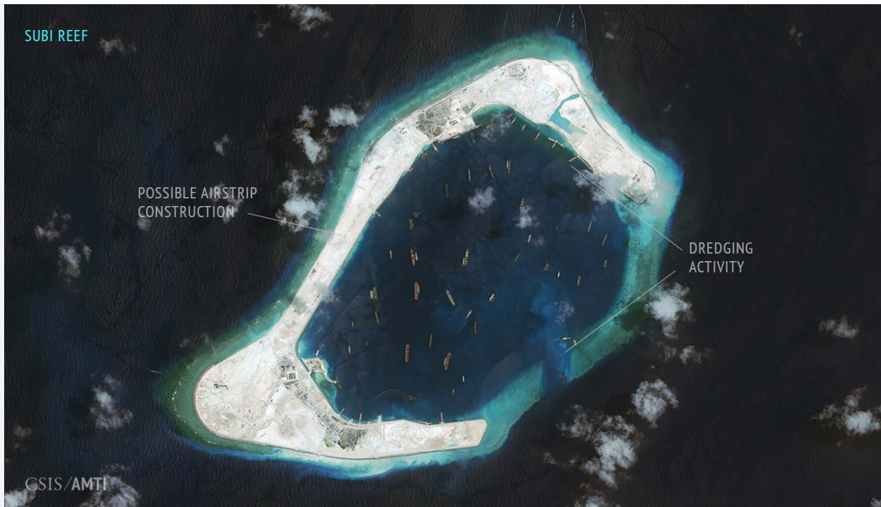
SUBI REEF. September 3, 2015. Possible runway construction is ongoing on the western rim of the reef. At the southeastern entrance, a dredger widens the access channel to the inner reef. To the northeast a second dredger completes land reclamation along the rim.
