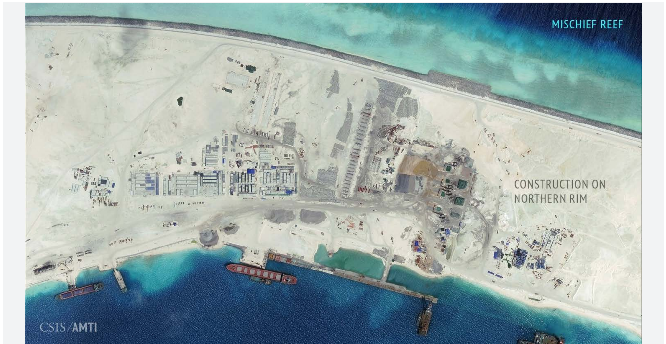
MISCHIEF REEF. September 8, 2015. Construction begins on Mischief Reef's northern rim. An area measuring 3,000+ meters in length has been cleared.
