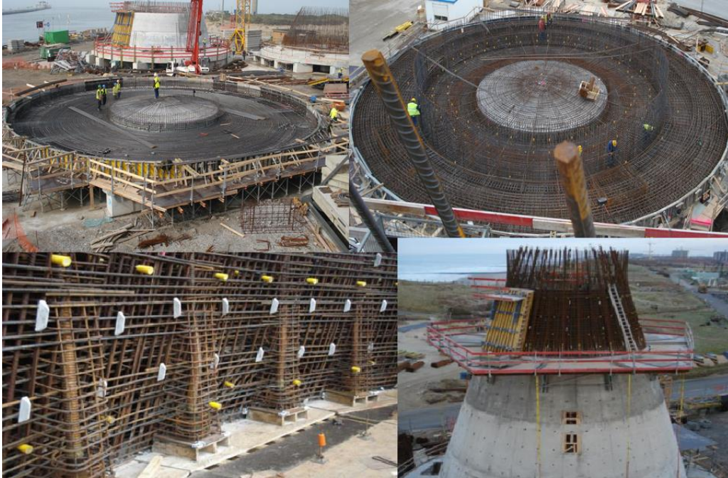
Figure 8-6: Gravity Foundation Production Facility
